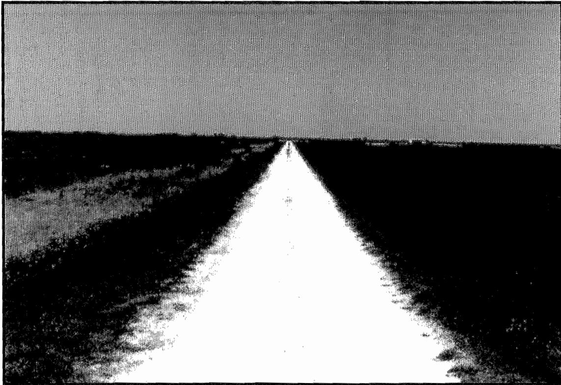
Levee 74-N, looking north, just south of the C-54 Retention Pump Station.
